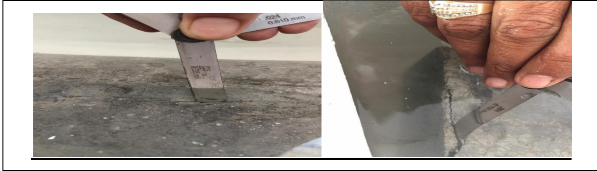
Figure: - 5.5.1 Crack measurement with Gauge meter.
